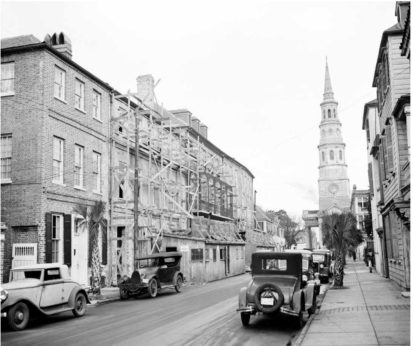
The Dock Street Theatre, with scaffolding on facade, at Church and Queen Streets in Charleston, S.C., is seen on January 20, 1937 as restoration nears completion. Phillips Episcopal Church, founded in 1620, is seen in background. Photo: AP Images
