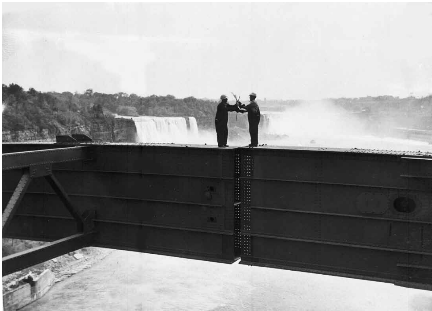
Two workmen, one from Canada and one from the United States, met, shook hands and exchanged flags on the center of the new Rainbow Bridge, over the Niagara Falls, May 1941. The 53 ton center iron arch of the bridge had been swung into place, leaving an 11-inch gap, seen between the two men, to be filled in later. (AP Photo)
