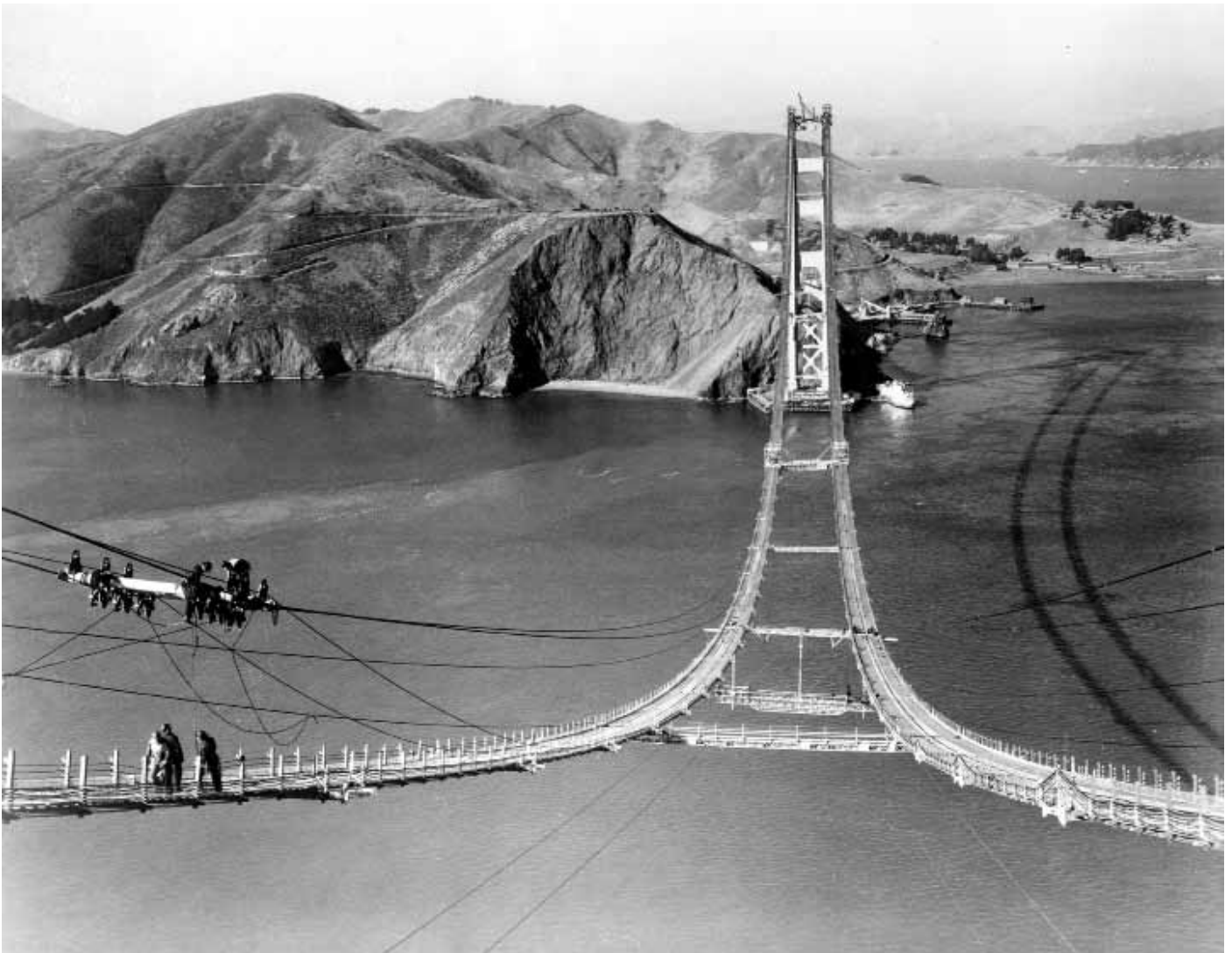
Workers complete the catwalks for the Golden Gate Bridge, spanning the Golden Gate Strait, prior to spinning the bridge cables during construction in San Francisco, October 25, 1935. (AP Photo)
