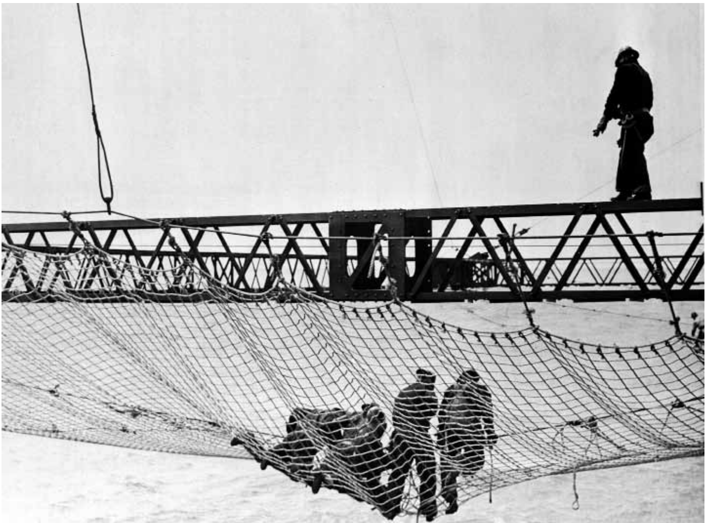
Workers install the first section of a huge safety net, at a cost of $98,000, that extended from shore to shore beneath the Golden Gate Bridge span during construction of the bridge in San Francisco, September 2, 1935. (AP Photo)
